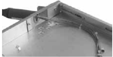
Distribution head outside the box with restricted fitting (sloped entry)
