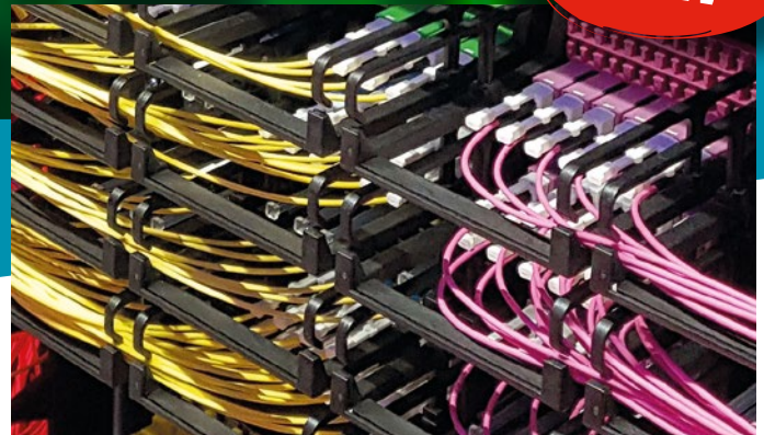
HIGH-DENSITY DATACENTER SOLUTION (HD-DCS)
